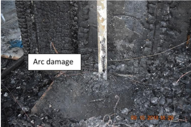
Image of the arcing damage at the base of the riser
