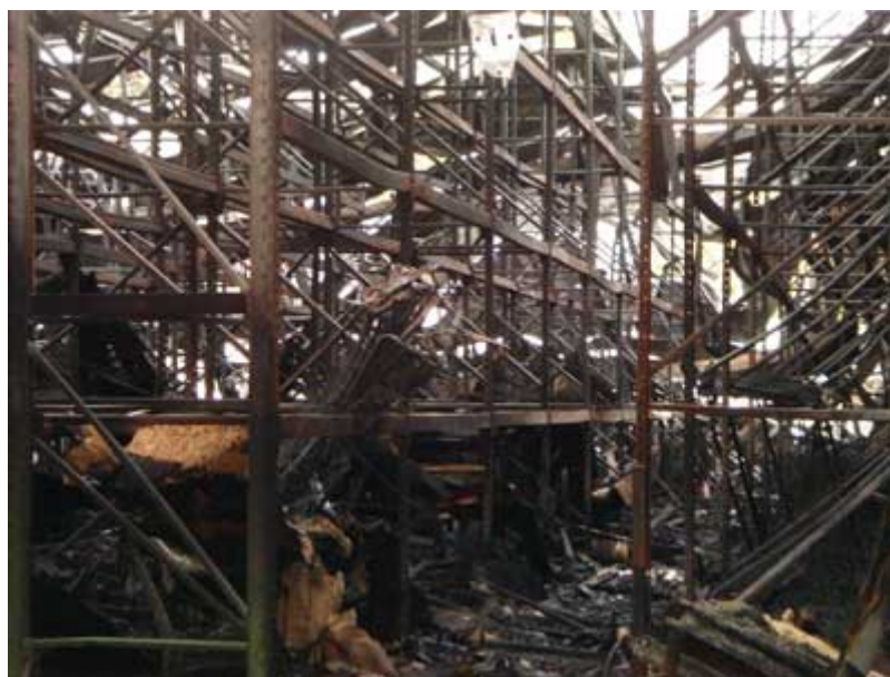
Photo 9. Storage racks in warehouse post fire. Storage racks were filled with various furniture and mattress items. Note the extent to which the storage racks filled the warehouse which gives an indication of the volume of merchandise and the fuel load inside the 15,600 square foot warehouse. The warehouse measured approximately 130 ft. by 120 ft. and was 29 ft from floor to roof.
